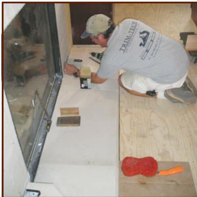
Fireplace that has been prepared for installation. And the installer is working on leveling and setting the hearth stones.
